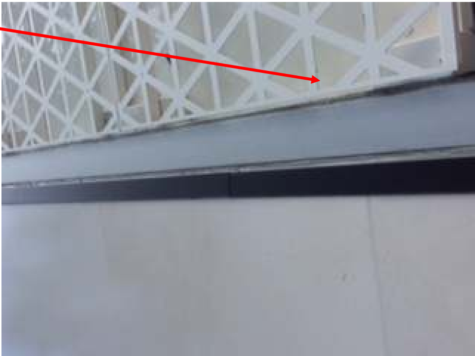
Metal trim does not line up
