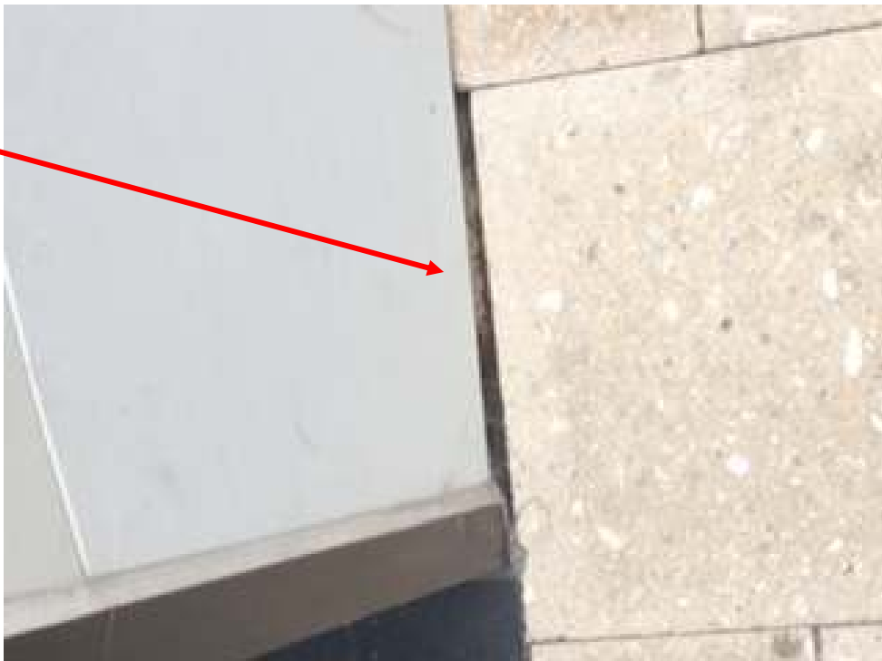
Improper placement of mall tile
