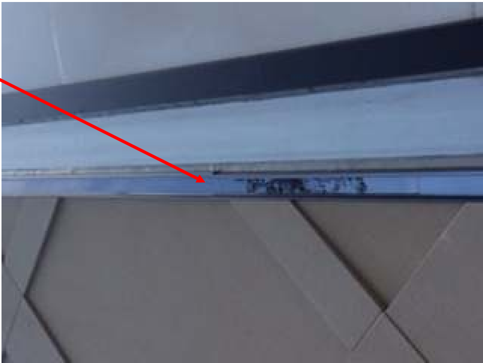
Metal does not line up on the vertical
