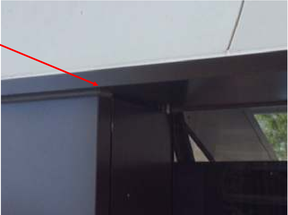
Metal closer not properly installed
