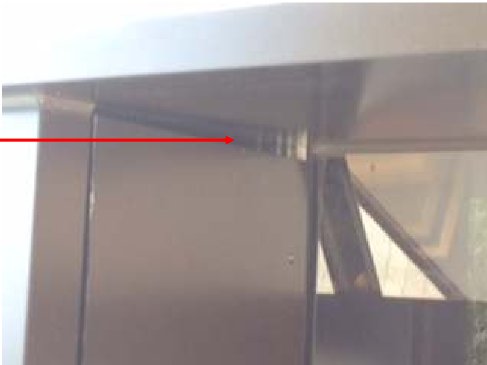
Metal closure not properly set
