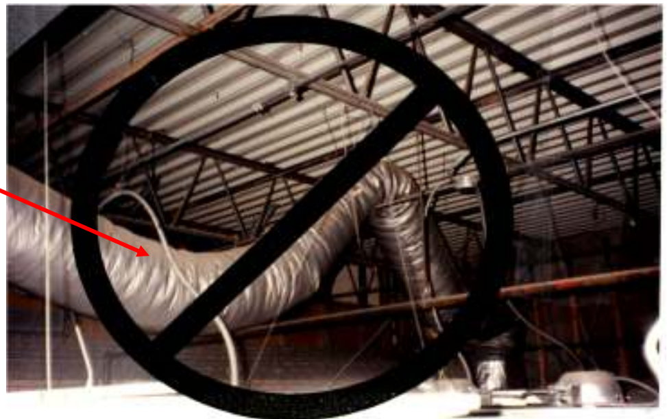
Length exceeds 5; Duct runs horizontal rather than vertical. Improperly supported.
