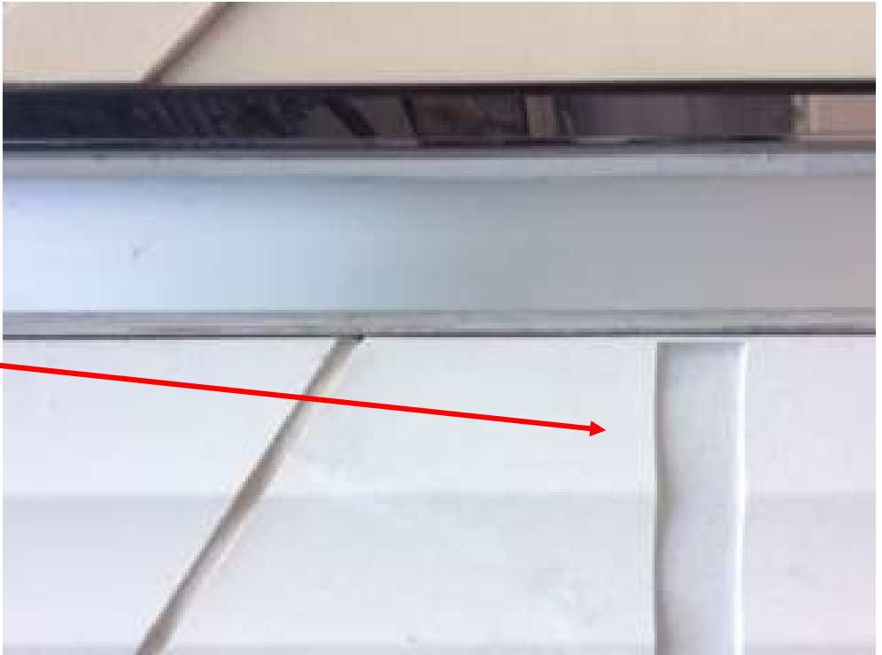
Poor workmanship on vertical caulk joint
