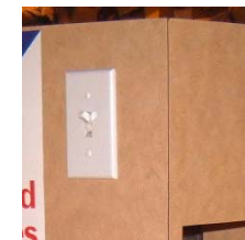
Exposed switches and plates.
