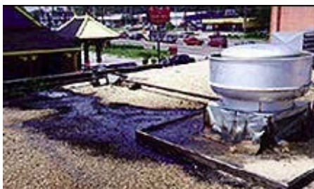
Roof Without Grease Guard Protection
