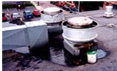
Roof Without Grease Guard Protection
